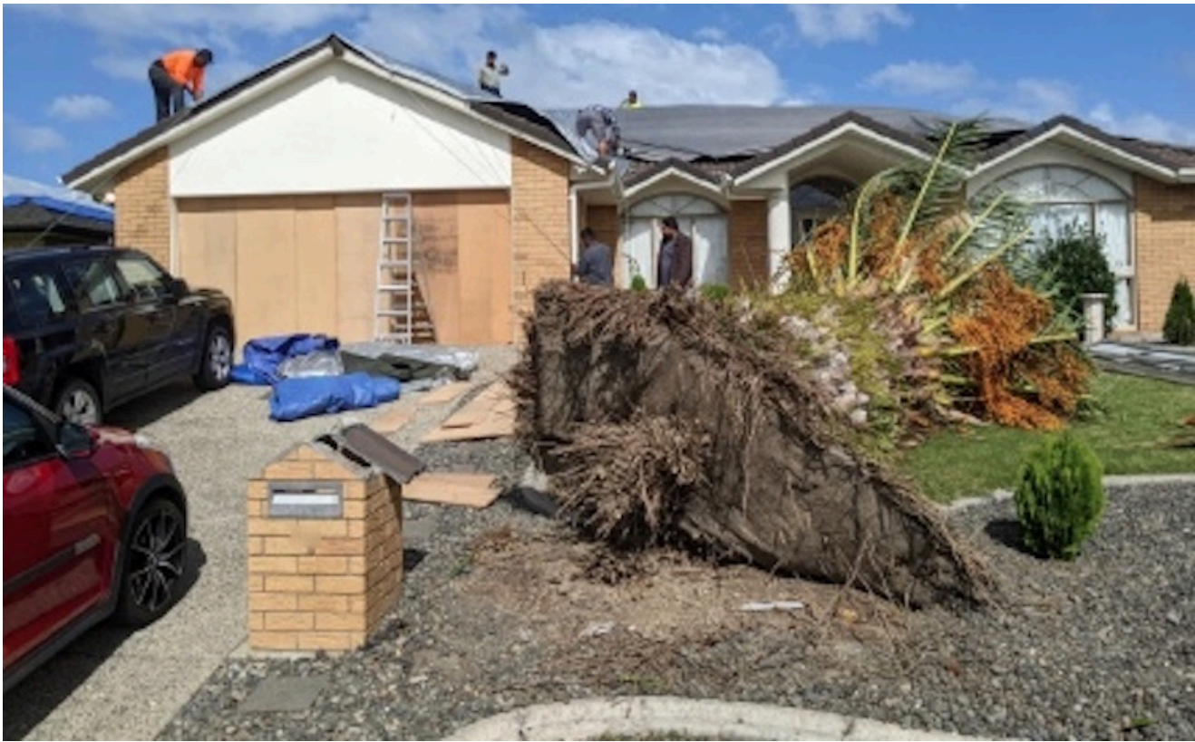
Tornado damaged house in Auckland. Credit: RNZ
